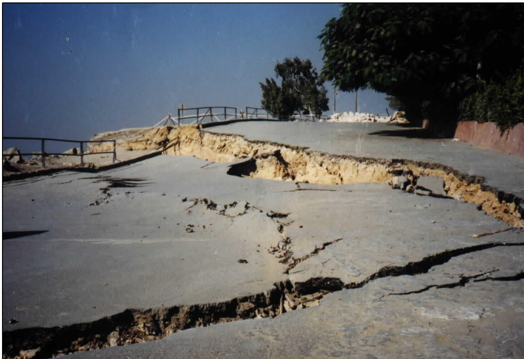
Figure 1-4: Soil failure (www.4isfge.org).
