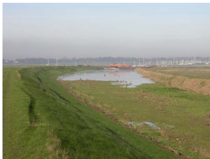
Maintenance dredged material is being pumped into containment bunds to create new salt-marsh (Wallasea, UK).
