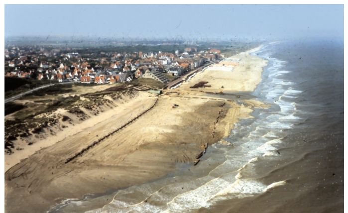
Figure 3: Profile nourishment in combination with reclamation of the subtidal (submerged) beach at De Haan Belgium for sustainable and integrated coastal defence
